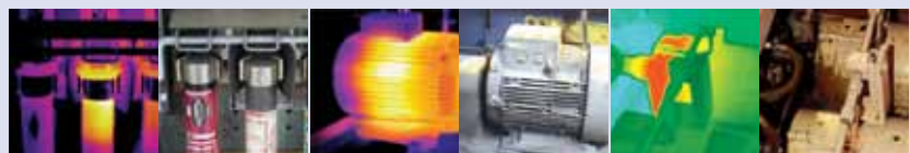
Electrical: Hot Fuses
